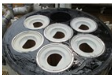
Natural Gas Plant Amine Unit – Bags To V-Max
